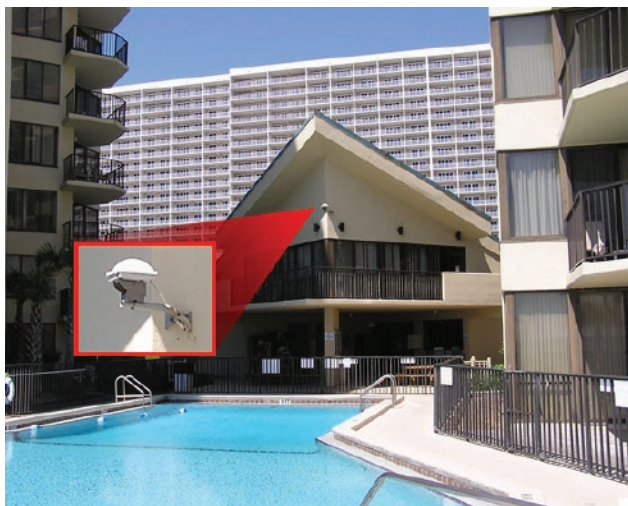
A ZoneFlex 2741 802.11g "root AP" mounted on the recreation building signals out to other mesh APs located on broadcast towers around the 5-acre property.
